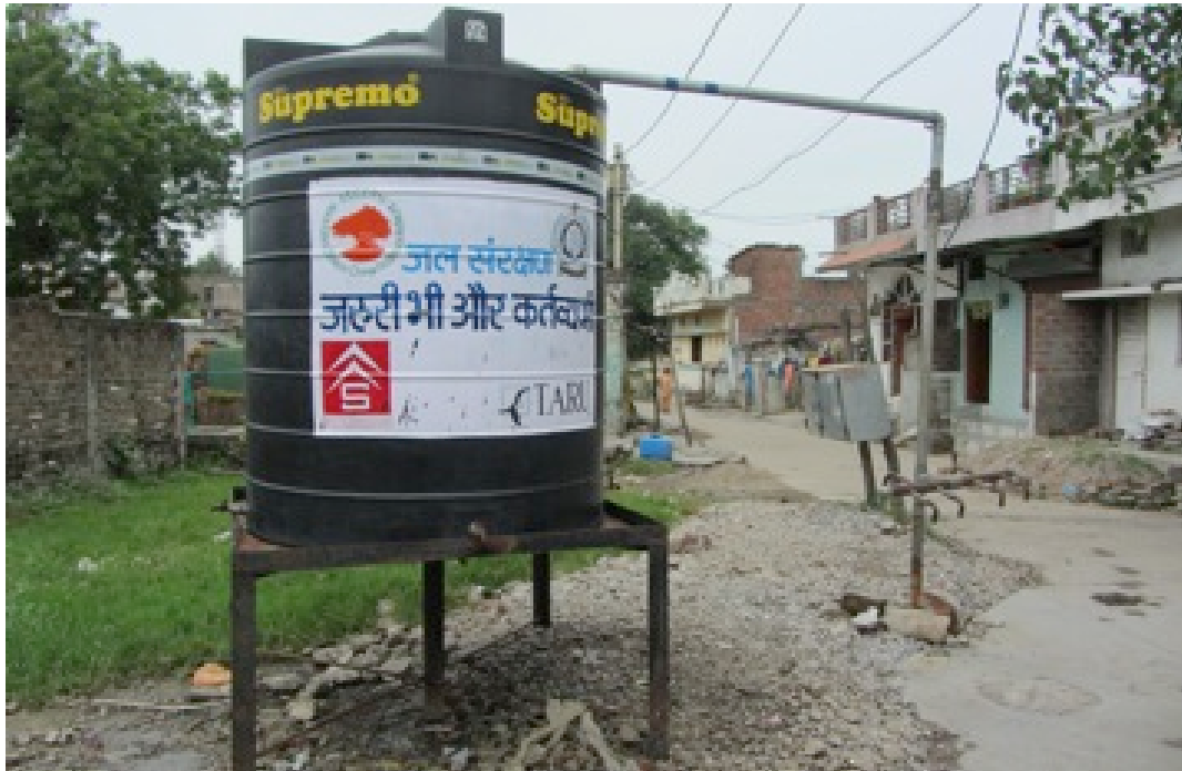
Figure 3. A water pumping station in Indore (photo taken by author)
