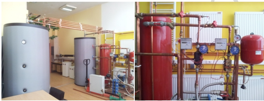
162 163 Fig. 3: Carried installation with tanks heat and cooling energy within the experimental demonstration of the 164 laboratory system.
