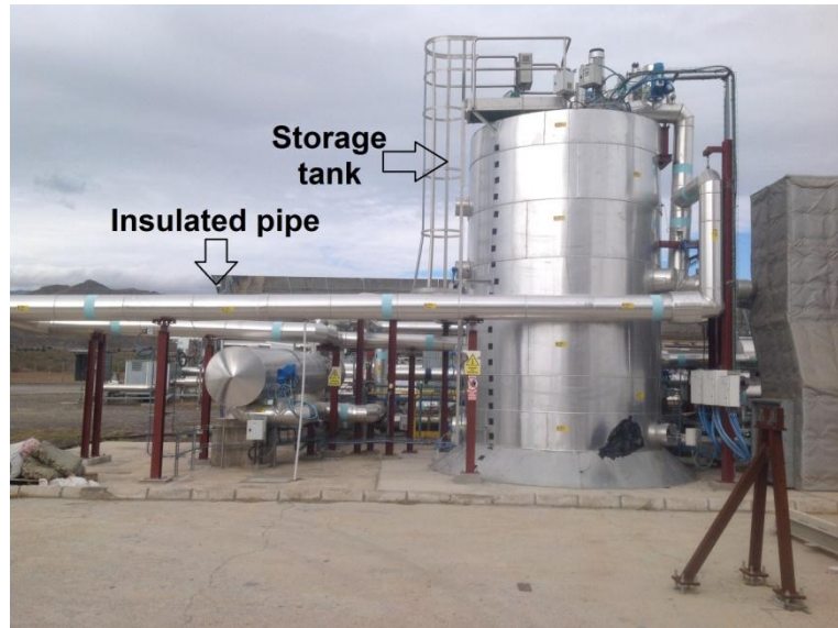
1 2 Figure 4: The photograph shows insulated pipelines and a molten salt storage tank at PSA, 3 Tabernas Desert, Spain. 4
