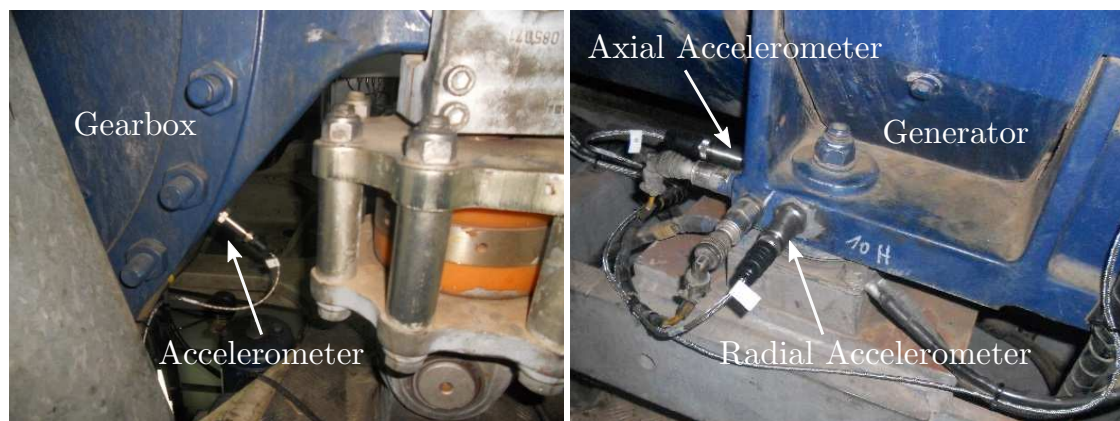
Figure 4. The radial vibration sensor installed near the planetary gear on the left and both axial and radial vibration sensors installed on the generator drive end on the right.
