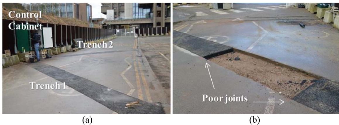
Figure 2: (a) The two reinstated trenches and (b) construction of the poor joints
