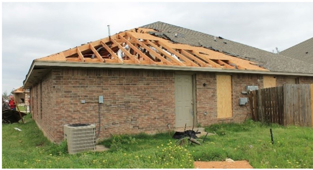
FIGURE 1 | Example of roof sheathing failure, corresponding to DOD-4 (image source: Dr. David Prevatt of University of Florida).
