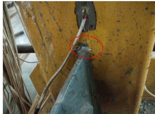
(f) Fracture near the top of gusset plate
