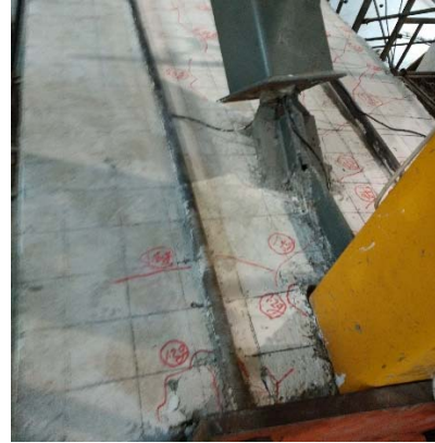
(b) Slab cracks near right column in the 1st story
