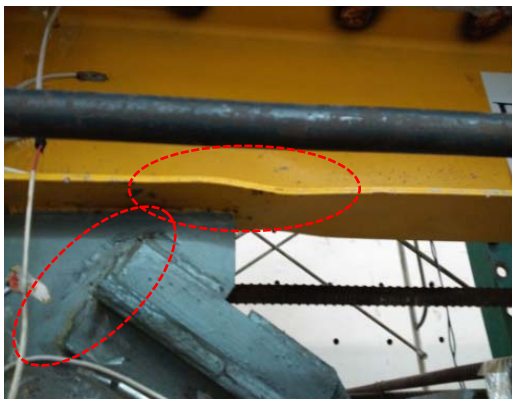
(e) Buckled beam bottom flange and gusset plate in the 1st story
