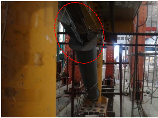
(a) Out-of-plane deformation of BRB in the 1st story
