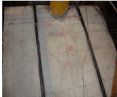
(b) Slab cracks near right column in the 1st story
