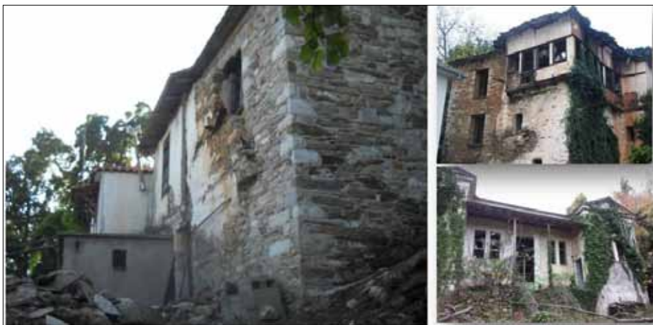
Fig. 6. Abandoned derelict properties
