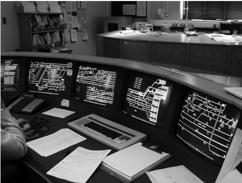
Figure 2. The signaller's workstation.
