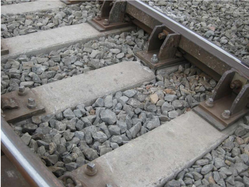
Fig. 4. Damage of concrete bearer (3.5-4m) underneath a v-crossing panel
