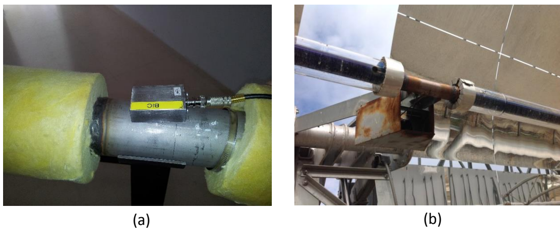
Figure 4. Detail of the junction of the collector tubes in the experimental platform (a) and in a real CSP in Almeria, Spain (b).
