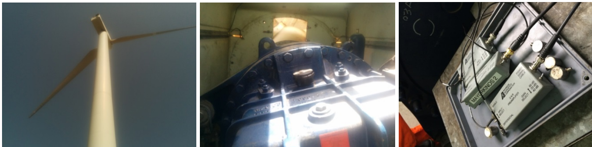
Figure 10: The 850 kW TERN Energy wind turbine gearbox instrumented in Crete together with the AE sensors and pre-amplifiers employed for its instrumentation.
