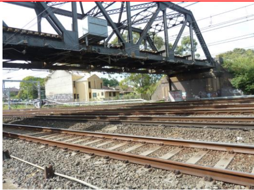
a) typical elevated transom bridge with vertical space constraints from roof trusses
