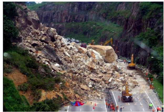
Figure 8: The Bukit Lanjan rockfall along the New Klang Valley Expressway, in November 2003, resulted in a six month closure of that particular stretch
