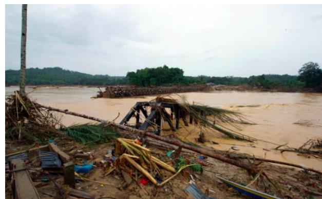
Figure 5: Malaysia East Coast Line railway bridge, which cross Nenggiri River in Kemubu, Kelantan had totally lost due to massive flood in December 2014.
