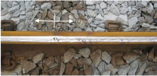
Fig. 7. Interface between SC rail and HH rail. The SC rail is squat free. Squats are visible at the weld and in the HH rail. High rail in transition to 932m radius curve [5].
