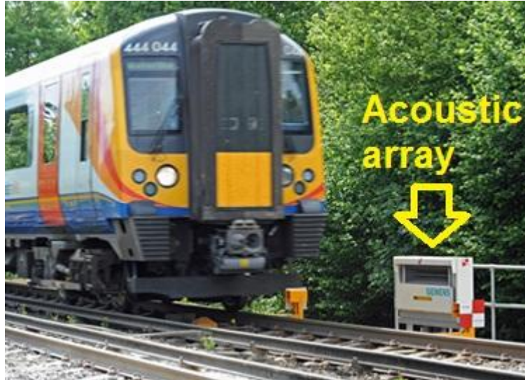
Figure 4: A RailBAM trackside acoustic array detector installed on the British rail network near London (the photograph is courtesy of SIEMENS).
