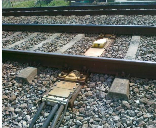
Figure 3: A Hot Axle Box Detector installed on the Portuguese rail network (REFER).
