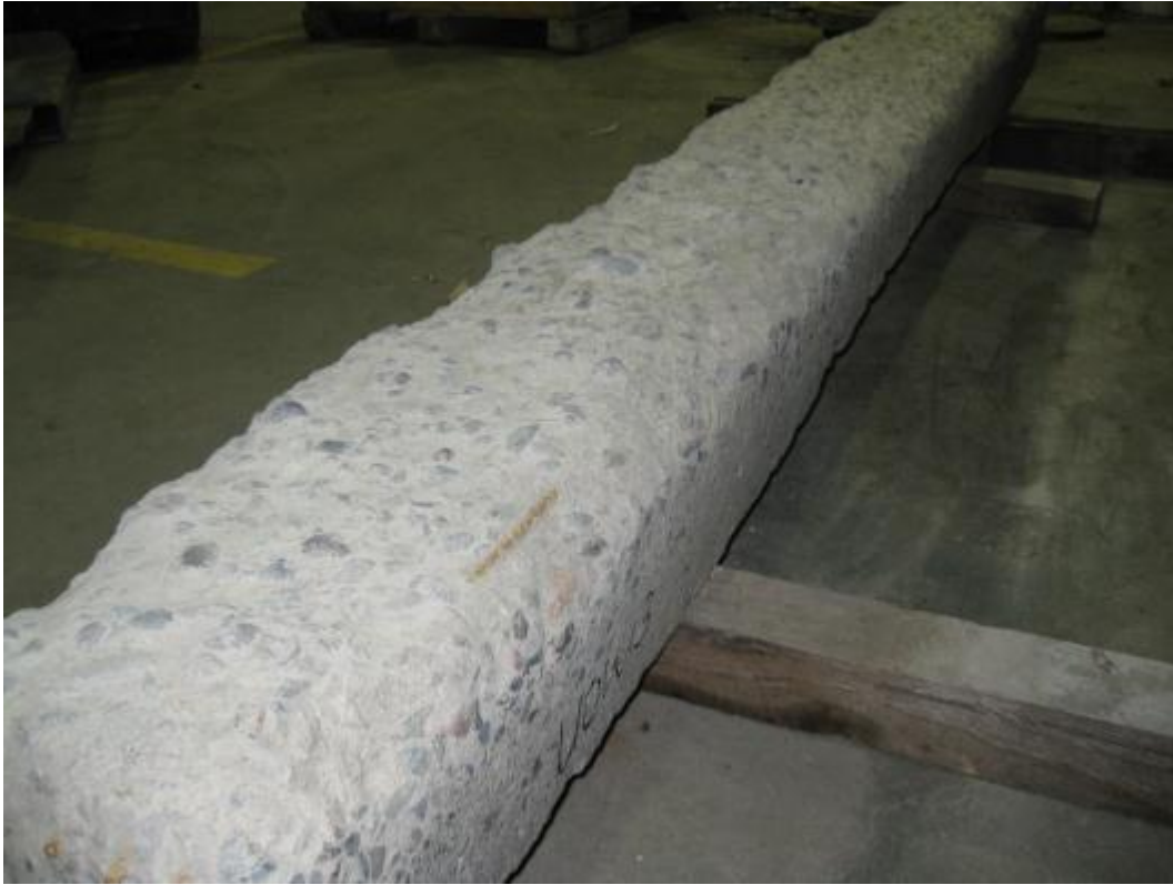
722 723 c) severe abrasion of the concrete cover at the bottom surface of sleeper UOW3, causing one of prestressing wires was 724 exposed 725
