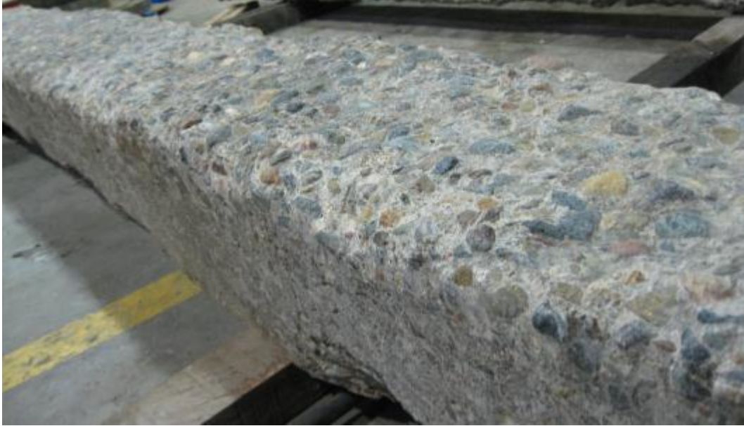
e) severe abrasion of the concrete cover at the bottom surface of sleeper UOW5
