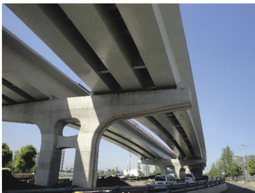
Figure 1. The typical OSD bridge selected for investigation (courtesy of Dr Junlin HENG).
