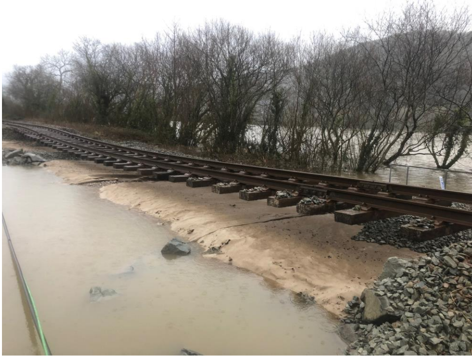
Figure 4. Washouts in 2020 leading to suspended track on the Conwy Valley Line (source: Network Rail)
