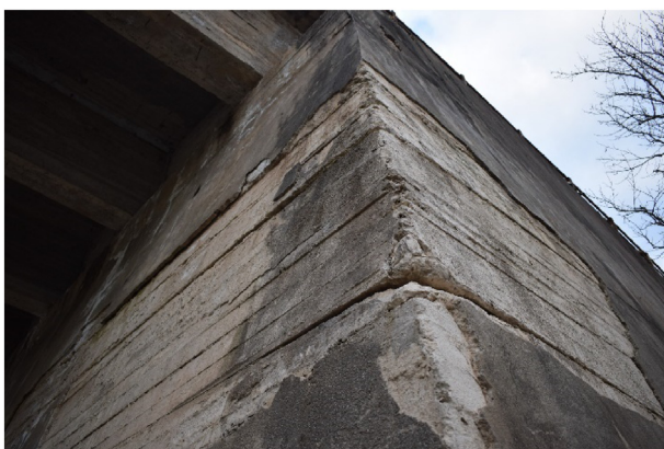
Fig. 9. Photo of the standing, east, abutment with evident relative displacements at the interfaces between concrete blocks, indicating that the joints act as weak zones.
