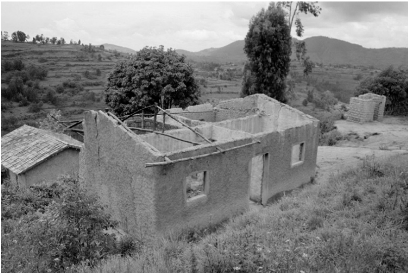
FIGURE 4.1 Destroyed house. Photo by the author.
