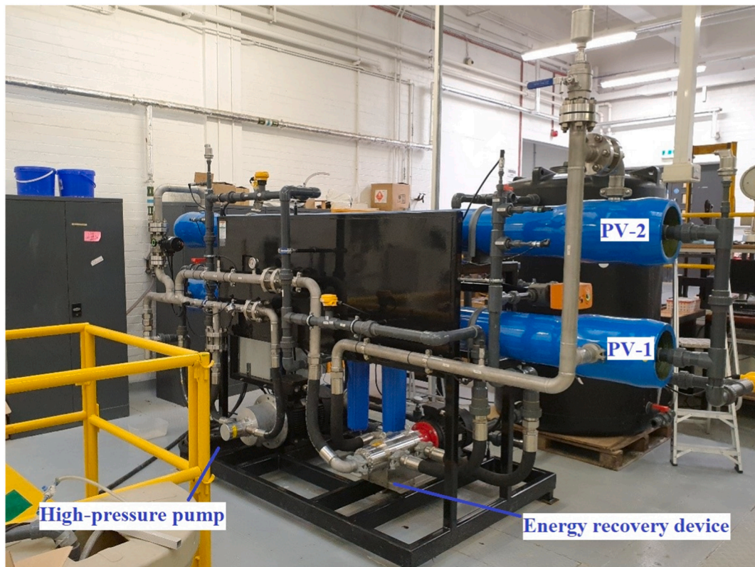
Fig. 1. RO system installed in the laboratory (front).
