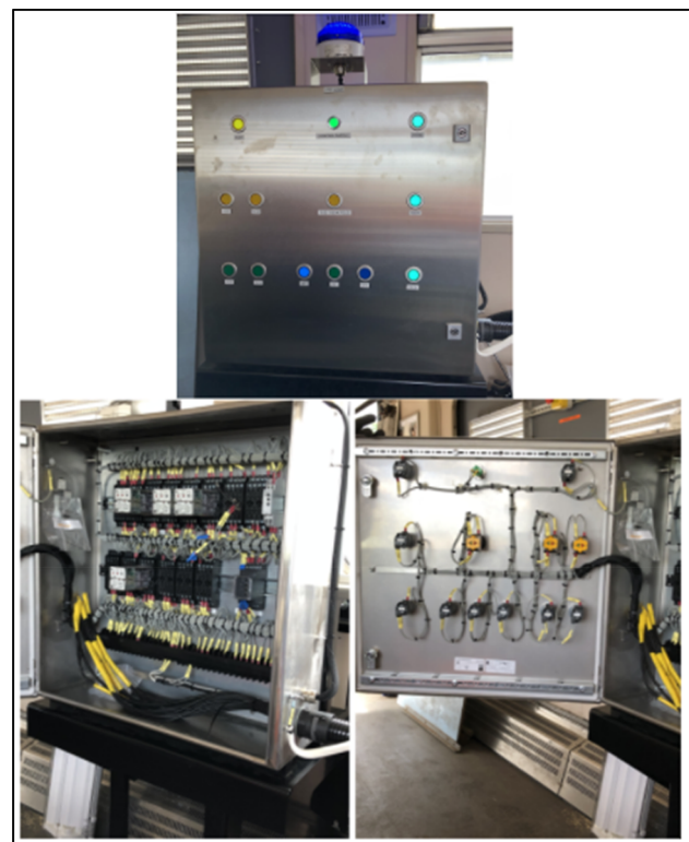
Fig. 6 Train control logic equipment, showing the exterior (above), and interior wiring (below)
