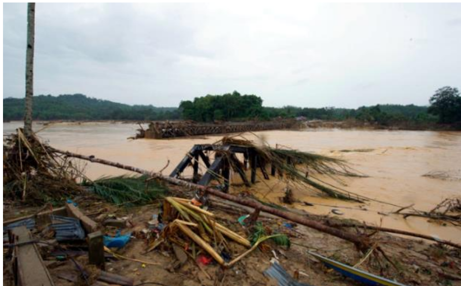
161 162 Fig. 3. Washaway of railway tracks occurred in Malaysia East Coast Line railway 163 bridge, which cross Nenggiri River in Kemubu, Kelantan had totally lost due to mas- 164 sive flood in December 2014. (Courtesy: Malaysian Department of Public Works)
