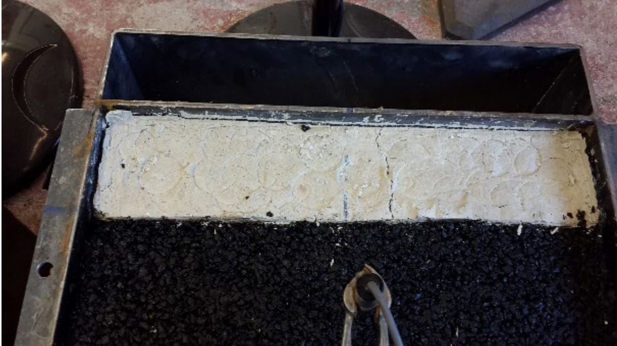
Figure 8 Illustration of a cross sectional crack on shoulder of a test section
