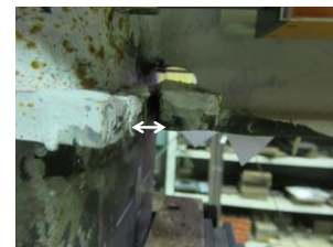
Retro. Specimen at 3.0% story drift: 20 mm separation of the bottom flange from the diaphragm edge
