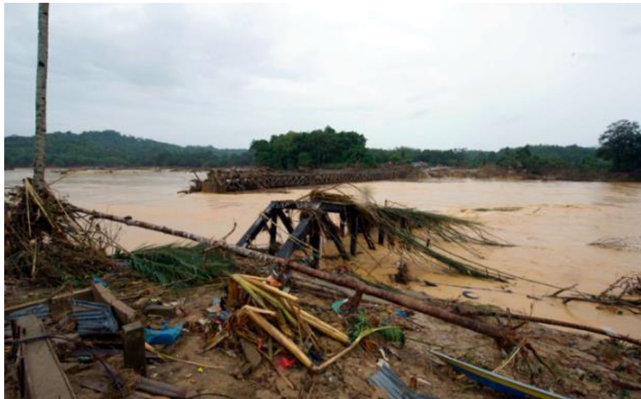
Fig. 3. Washway of railway tracks occurred in Malaysia East Coast Line railway bridge, which cross Nenggiri River in Kemubu, Kelantan had totally lost due to massive flood in December 2014. (Courtesy: Malaysian Department of Public Works)
