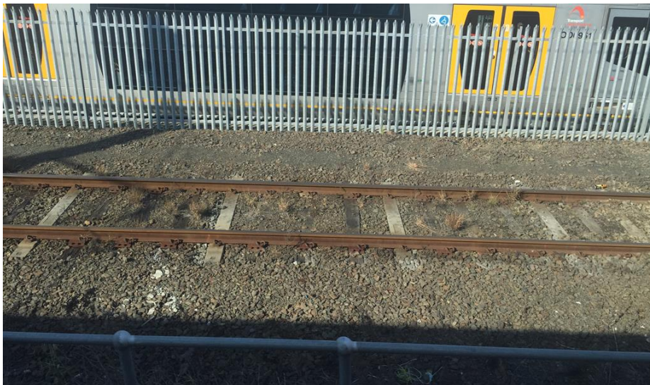
Fig. 2. Example of 1 in 4 interspersed tracks (1 concrete sleeper after 3 timber sleepers – a set of four)
