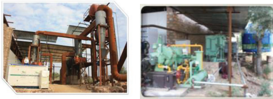
Fig. 4: Biomass Boiler, Turbine and VAM Set Up
